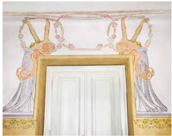
13. Art nouveau painting in Villa Poljanska 97 after restoration interventions, photo by Tjaša Pristov, 2014
