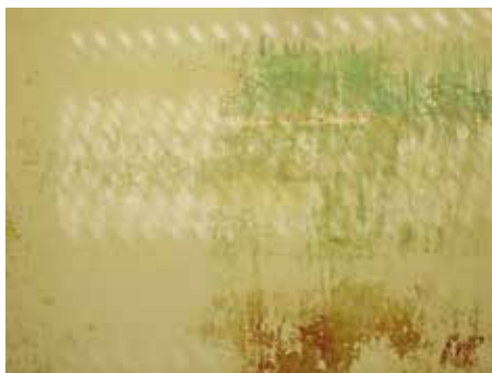
9. Deteriorated painting, photo by Heli Tuksam, 2014
