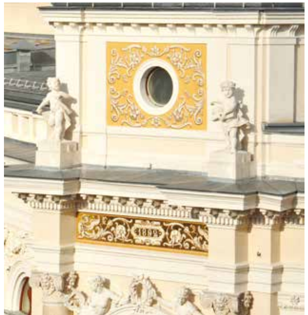
14. Paintings on the tower and the frieze of the south-eastern part of the building after the completion of restoration interventions, photo by Tjaša Pristov, 2010
