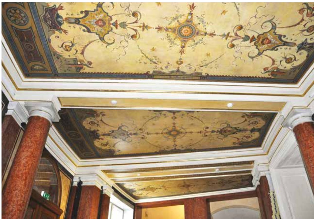
11. View of part of the ceiling in the lobby after the completion of restoration interventions, photo by Tjaša Pristov, 2010
