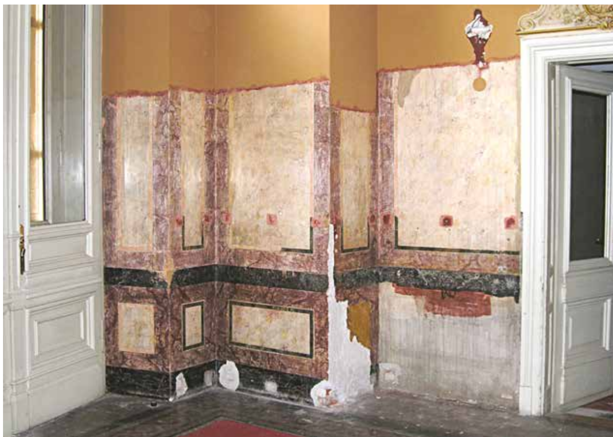
3. The uncovering of stucco-lustro on the southern wall of the foyer, photo by Tjaša Pristov, 2009
