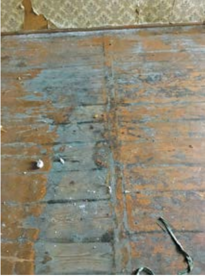
14 A. A fragment of the authentic flooring before restoration. Photo by Vincas Brezgys, 2017
